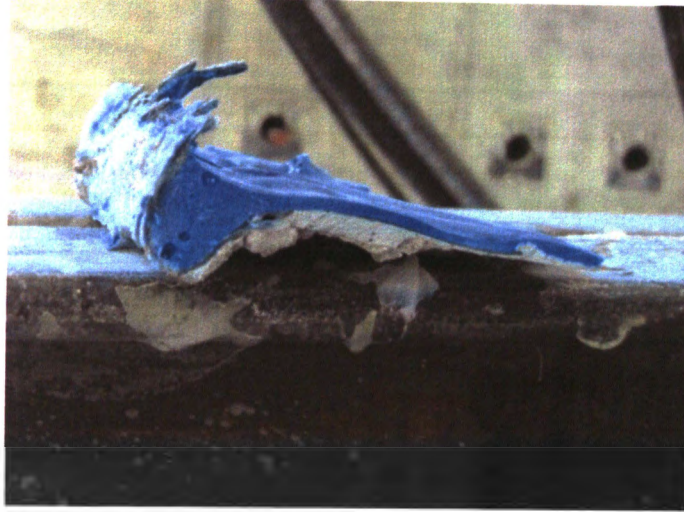
Figure 5.33. Failed U-Anchor After Removal From Groove
