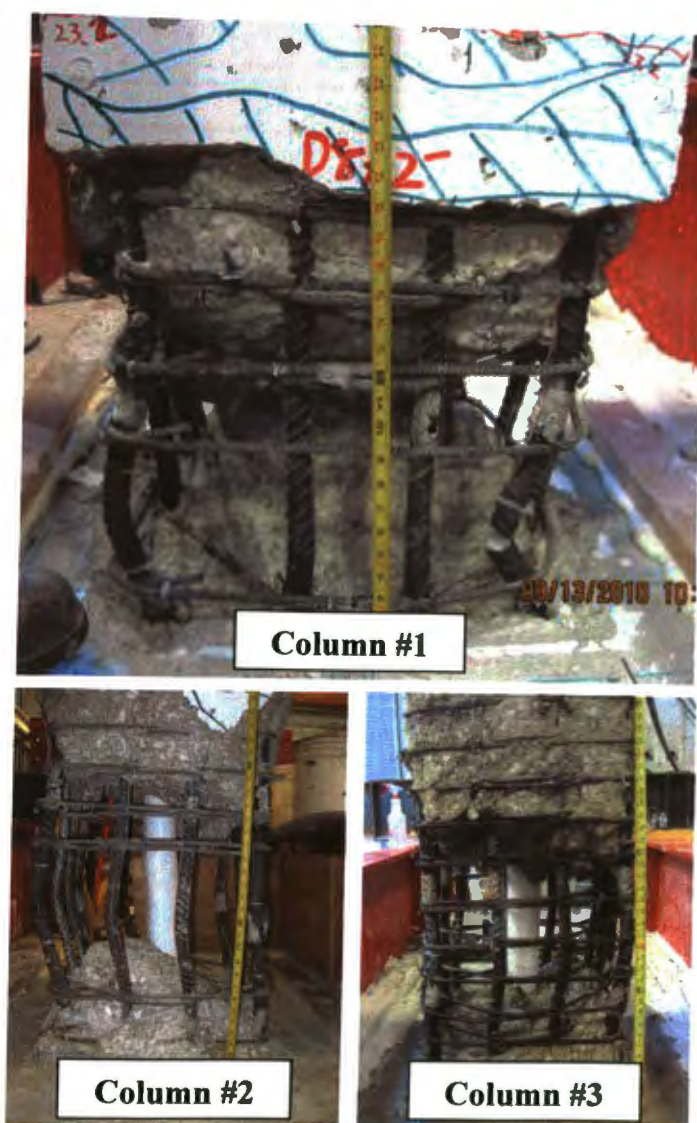
Figure 4.16. Columns After Removal of Loose Concrete
