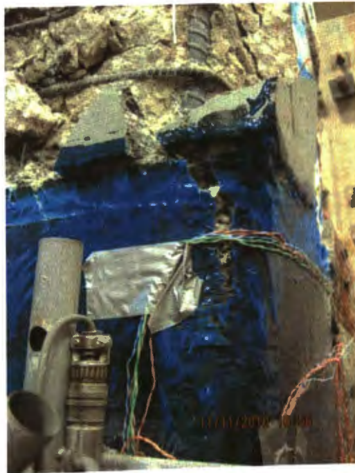
Figure 5.9. Rupture of Transverse CFRP on Southwest Corner of Column #3
